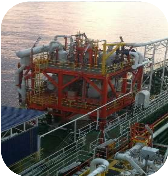
SEP-ISYS™ EWT installed on FSU Nautica
